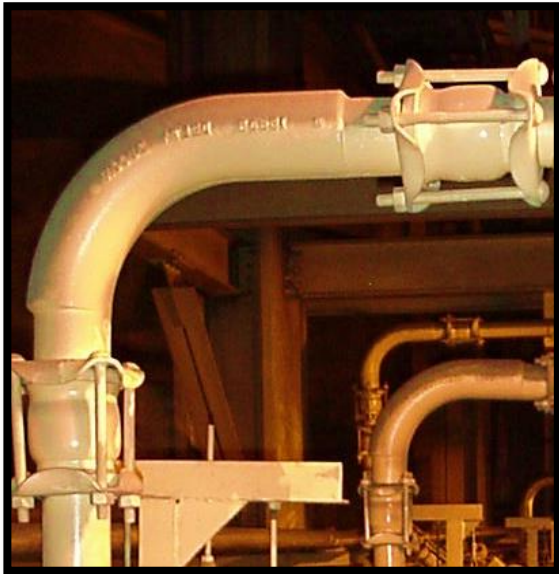
PWERMA/flo Conveying Piping
